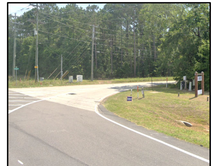
The missing yield sign on US 17 for northbound turning right onto Seewee Road.
